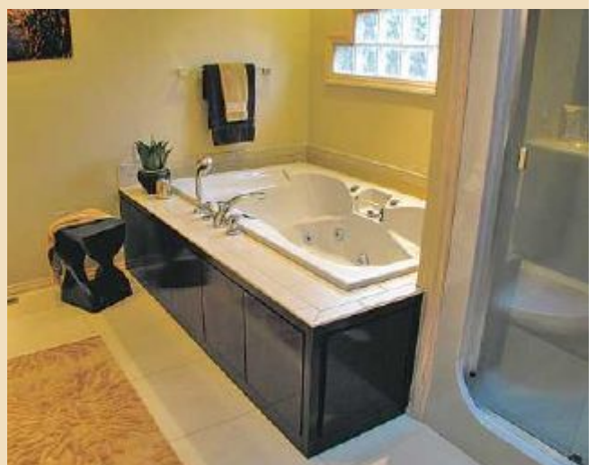
The bathtub stayed in place, but the old tiling was replaced by sleek cabinets that coordinate with the new vanity. Access panels to the plumbing are disguised beneath the cabinetry. Photo by Carrol Krause
